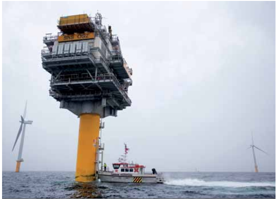
With all the foundations in place, substations positioned and wind turbines being progressively installed, the wind farm is taking shape.
